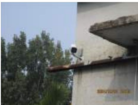
CCTV System (CCTV Camera)
